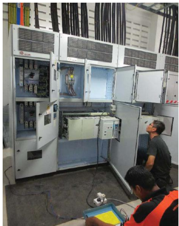
M1 Data Centre Main Switch Board Testing
